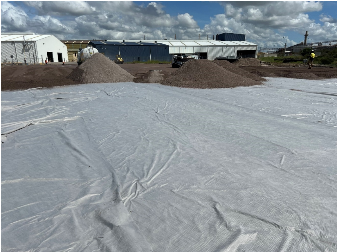
Photograph 1: Grey BIDIM A34G laid over lead and zinc impacted soil in the truck parking area
